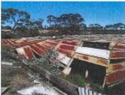
Ajana Dam with deteriorating corrugated metal covering
