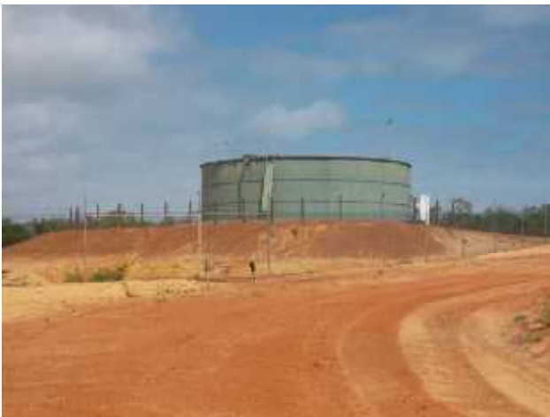
Photograph 3 – View of Water Corporation town water supply infrastructure located central on subject site.
