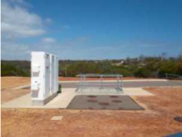
Photograph 5 – View of pump infrastructure located off George Grey Drive in the north west of the subject site.
